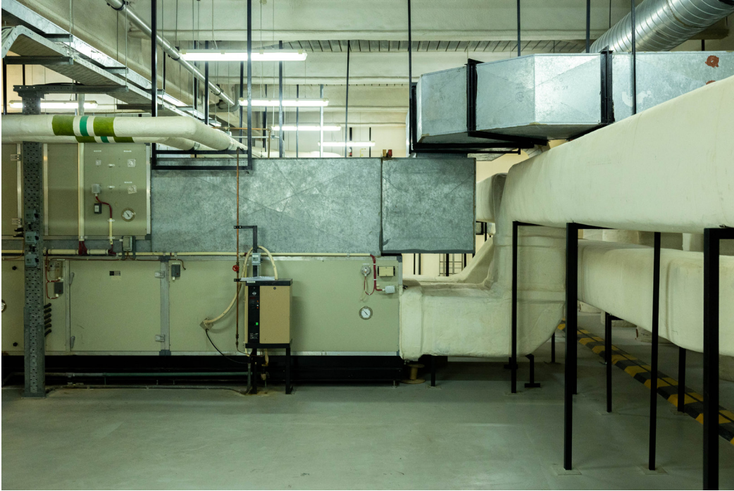
Fig. 2. Often out of sight, these plant rooms are the heart of Bahrain's National Museum. They gather ducts carrying fresh outdoor air into air handling units where the air is cooled and dispersed into the halls and galleries. Photographed by Hussain Al Mosawi.
